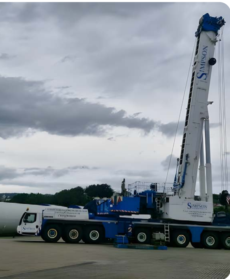
Turbine components, Lairg II
